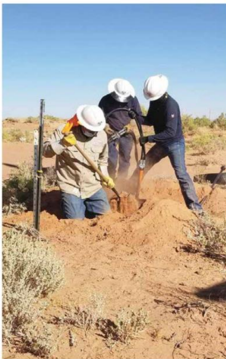
COURTESY PHOTO | NAVAJO TRIBAL UTILITY AUTHORITY
